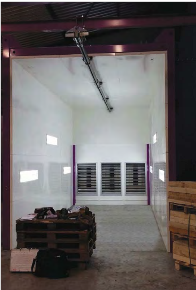
View from the inside of the paint booth with the integrated wall
